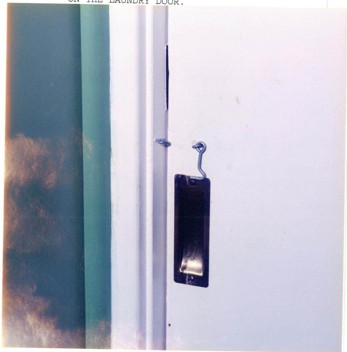
32. VIEW SHOWING THE UNLATCHED HOOK AND EYE ON THE LAUNDRY DOOR.
